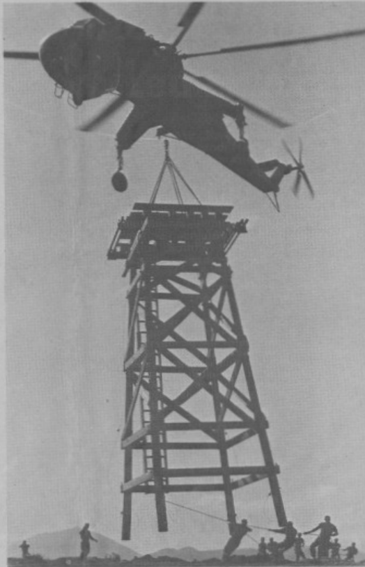
CRANE STRAIN —With a Sky Crane chopper doing the heavy work, Paratroopers from the 3rd Brigade guide a water tower support to its new resting place on a hill at Camp Evans. (Photo by Sgt. Jerry Ghearing)
