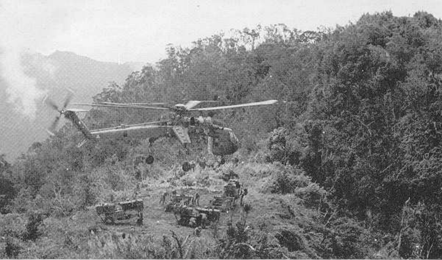
CH-54 "Flying Crane" drops a bulldozer blade on a newly cut landing zone on the Bach Ma. From this LZ the earth moving equipment expands the cleared area outward, forming the foundation of the fire base.
