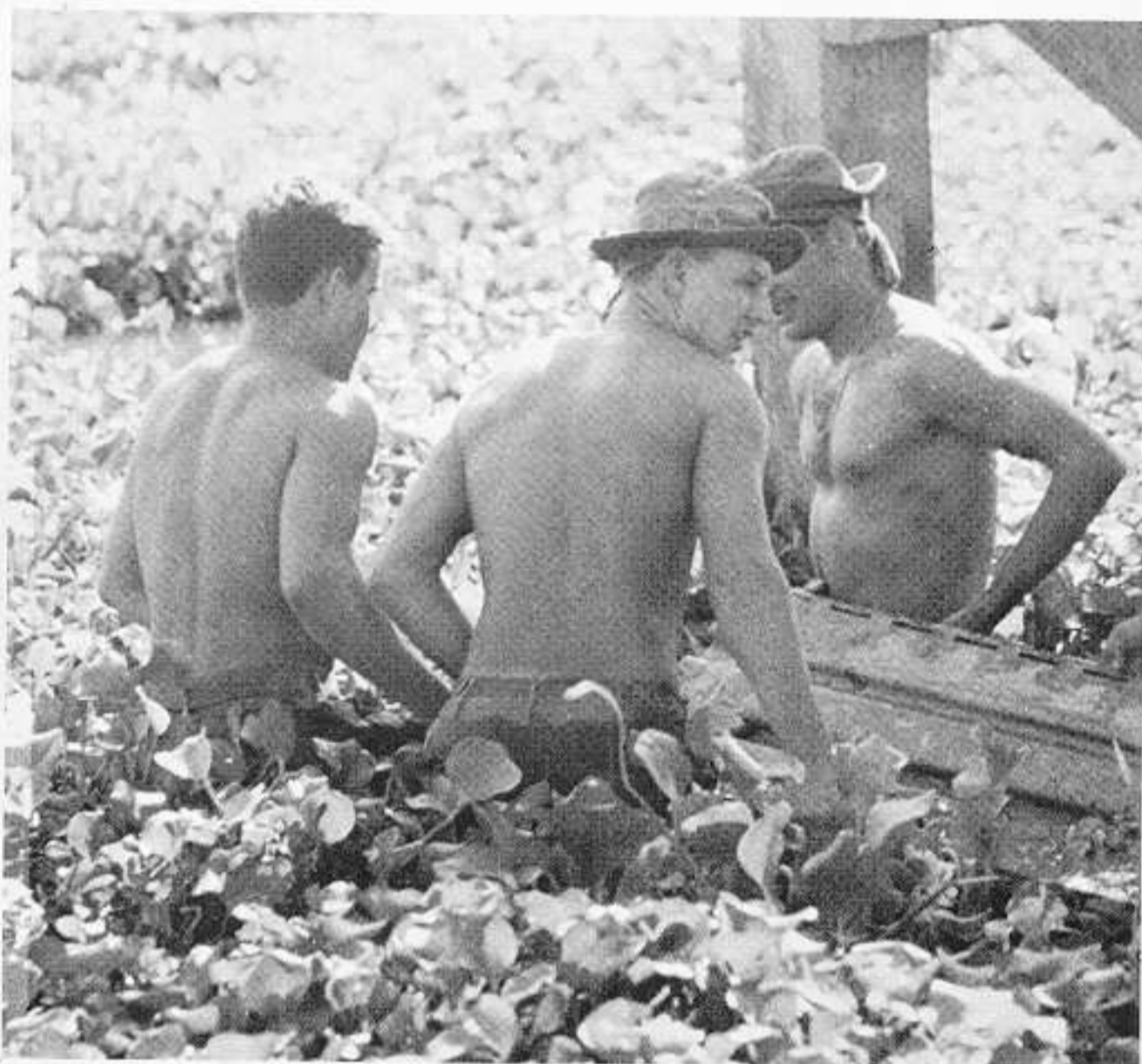
Work continues as the bridge, which will open farmlands to markets in Hue and Phu Bai nears completion.
