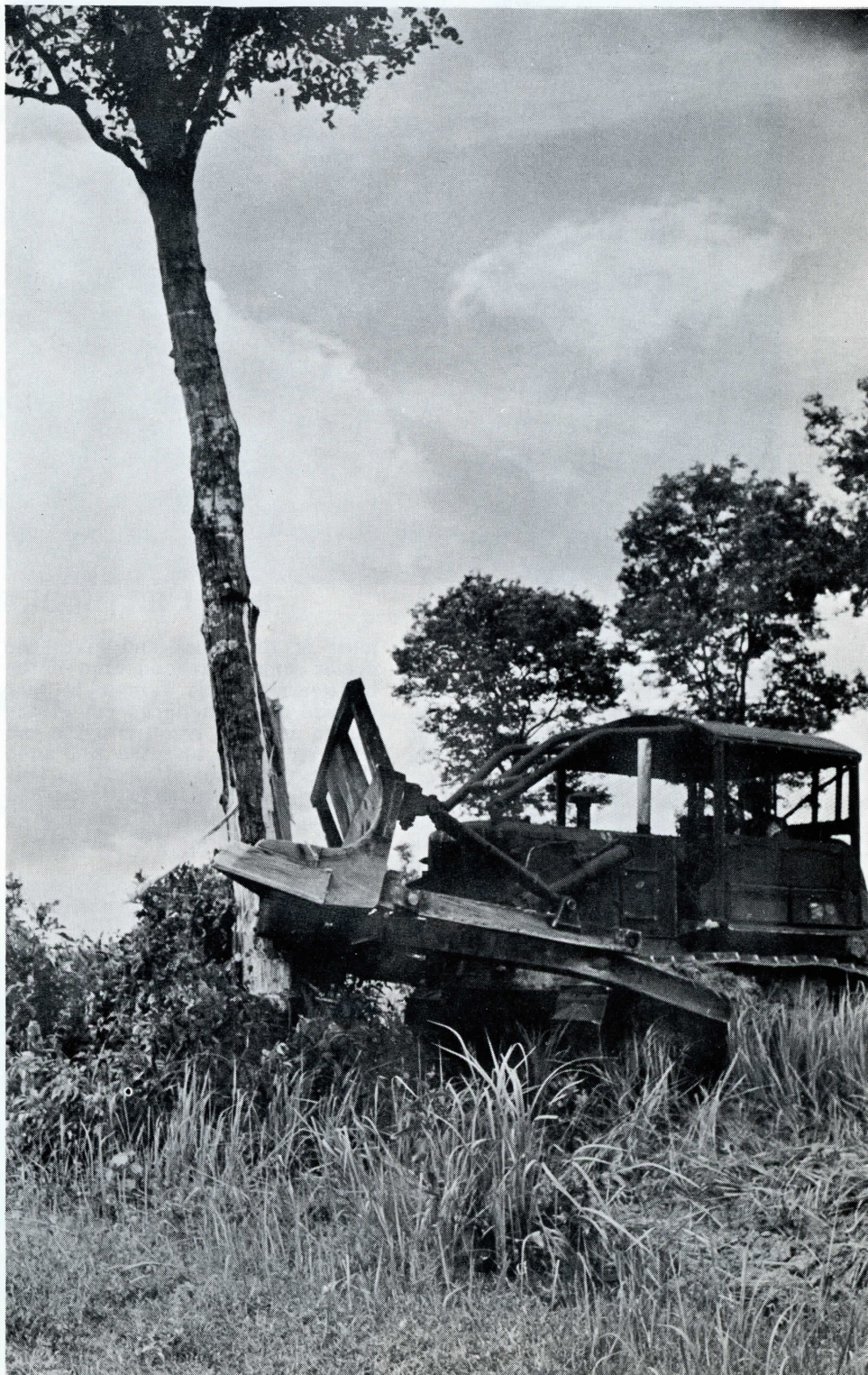
The stinger has split the tree and the operator attacks it with the main part of the blade. The tree is doomed and the enemy exposed
